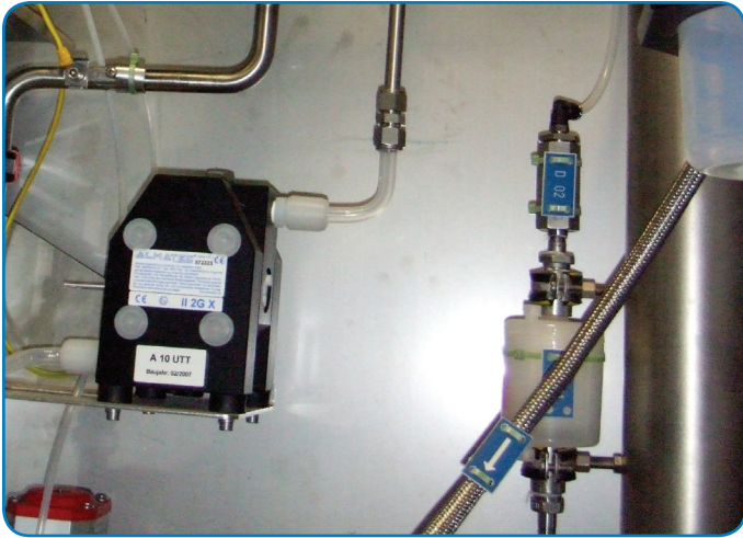
Pumps with conductive materials help chemical plants avoid electrostatic discharge, one of the greatest hazards when handling dangerous chemicals.
